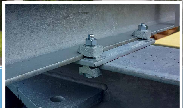
Girder Clamps connect the steel framework
