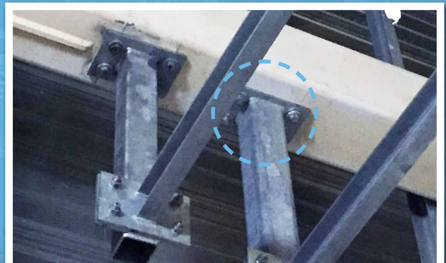
Hollo-Bolts used to connect pipe supports
